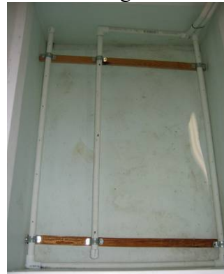
Interior of a standard 1,000 lb tote converted to a chiller tote by Doug Drum of Indian Valley Meats, at a cost of less than $50 for tubing and connectors.
